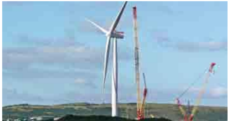
Siemens SWT-6.0-154 The long-bladed prototype is sited onshore at a test site in Scotland
